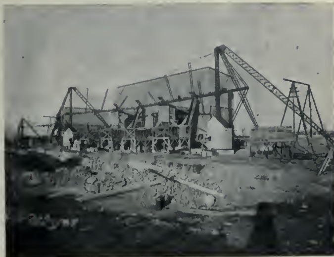
T. A. Morrison & Company's crushing plant. Cut of quarry shown on page 569
